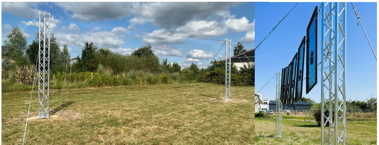
Figure 6. left side: Impression during construction phase; without PV modules; right side: first preliminary installation of the first row of modules.
