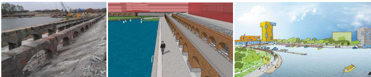
Images 13, 14 and 15: The construction of the quay wall at the Hout Dock, and two futuristic views (City of Ghent archives and sogent)
